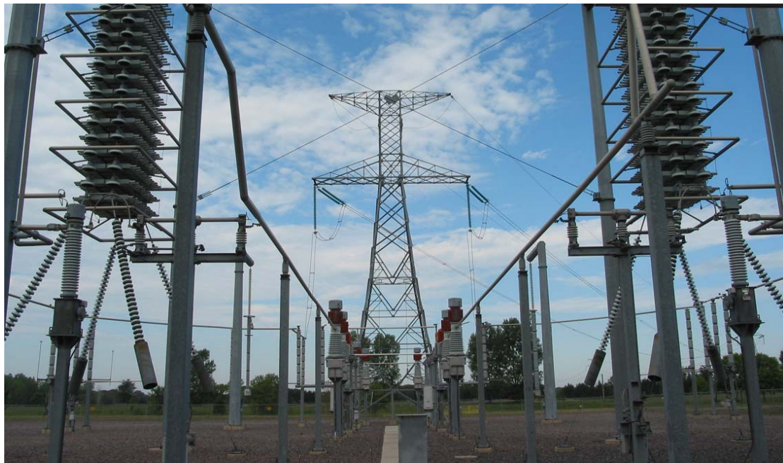
An HVDC converter station
