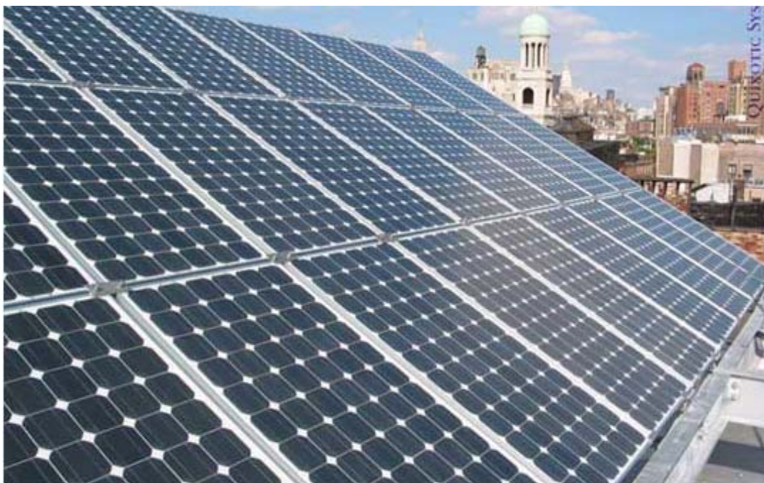
A rooftop PV installation
